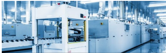
Control Systems PLC, DCS, HMIs, SCADA
